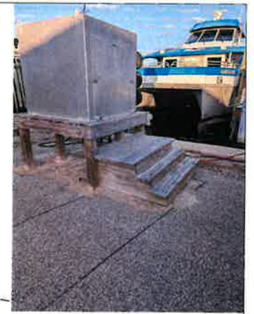
PHOTO 1 - EXISTING WATER BOX
